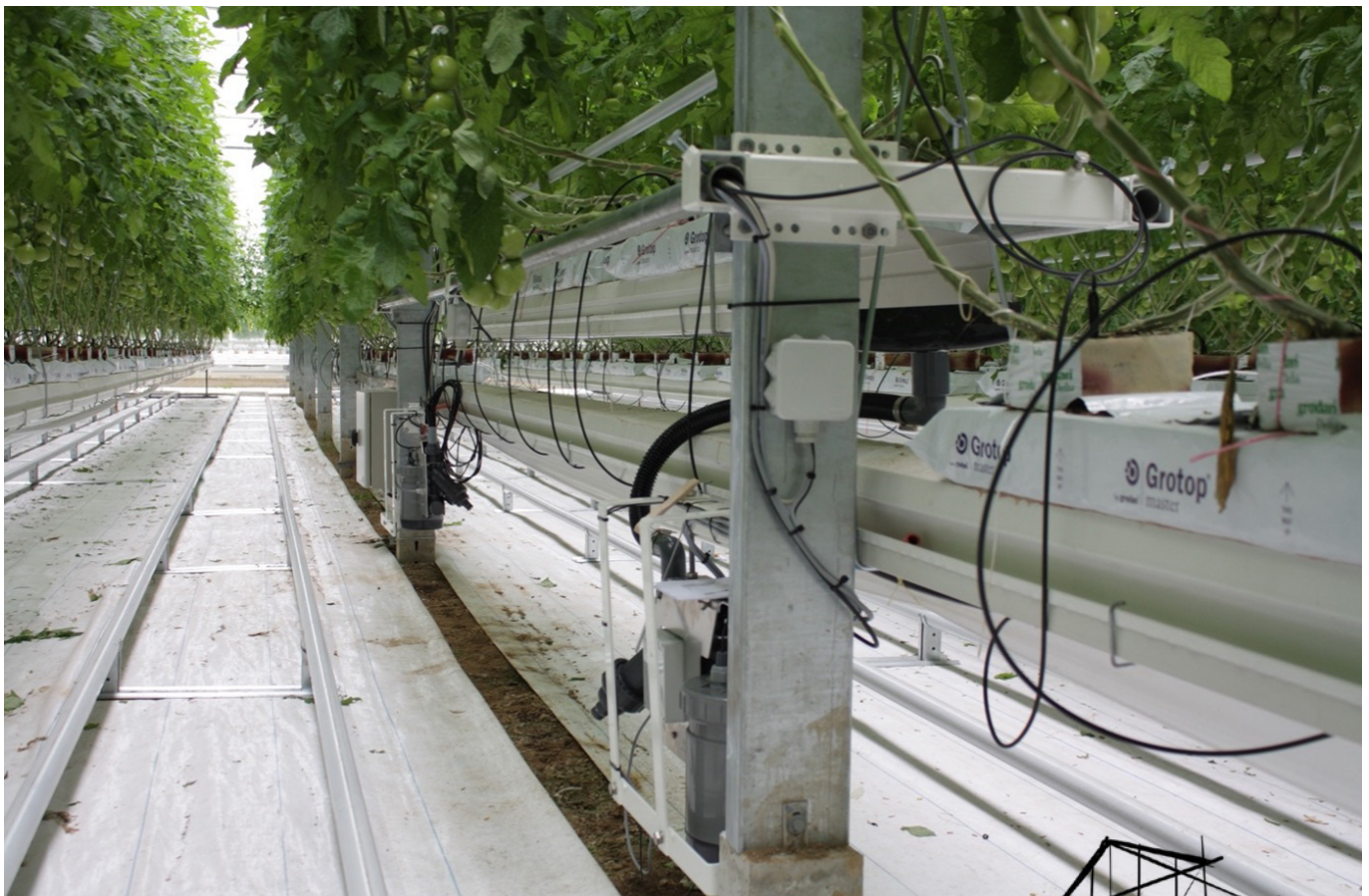
> Figure: Systems like ProDrain from Ridder interpret information from plant sensors to give insights into aspects such as transpiration.
